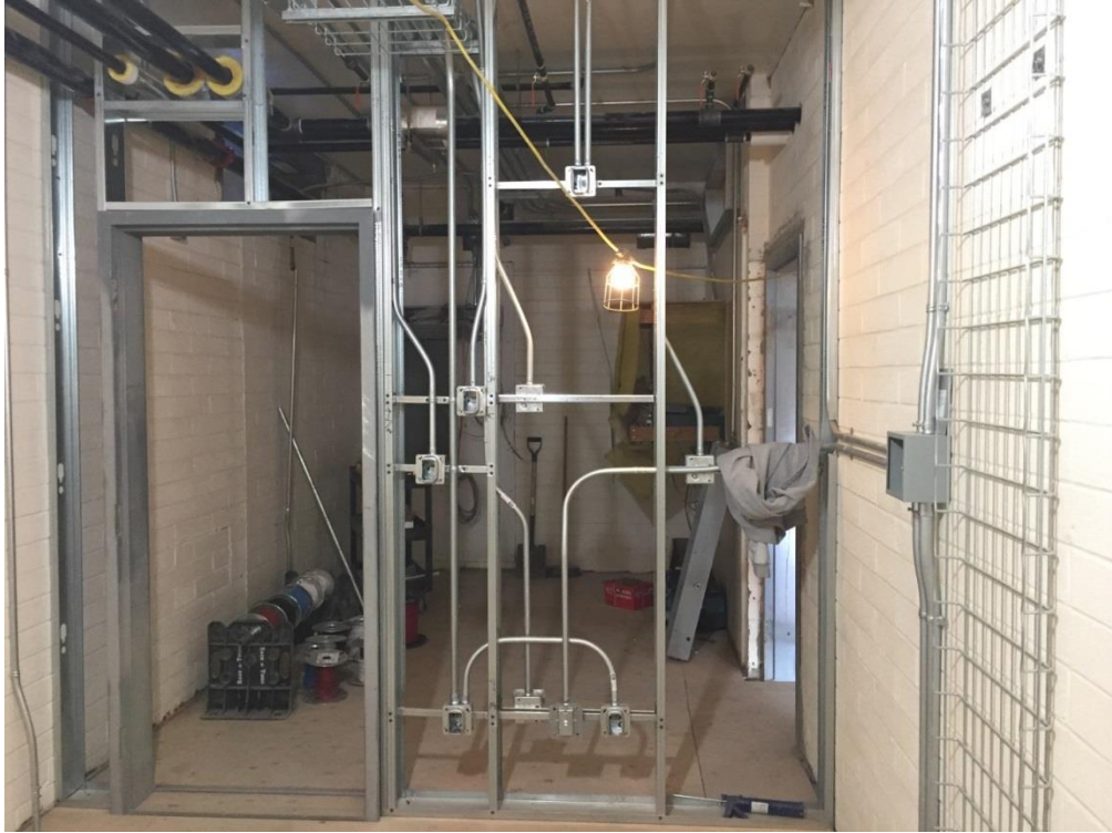
Future home of the data / server room
