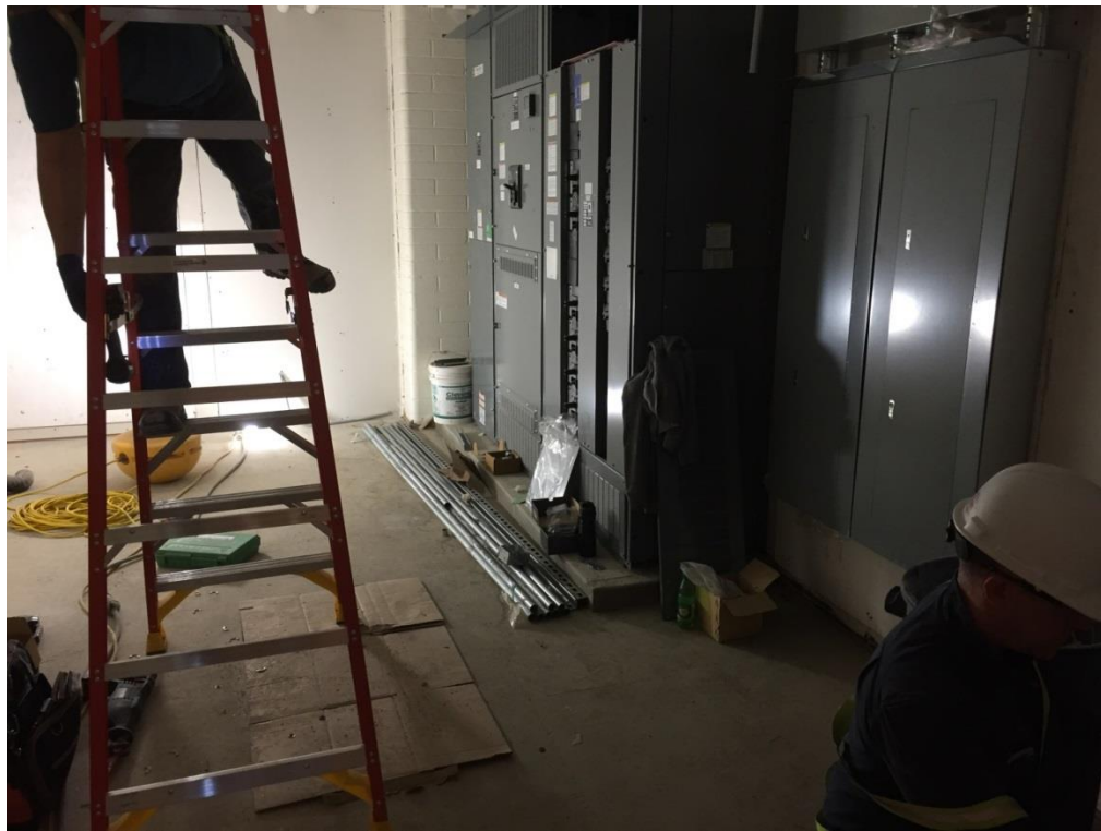
New main distribution panel and subpanels
