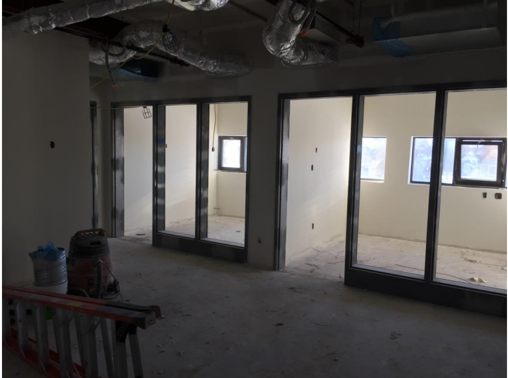
Example of the framing of office space upstairs in the School Division Finance area
