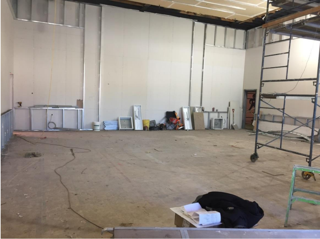
Council Chamber/Board room shows boarding finishes and architectural framing to support final finishes
