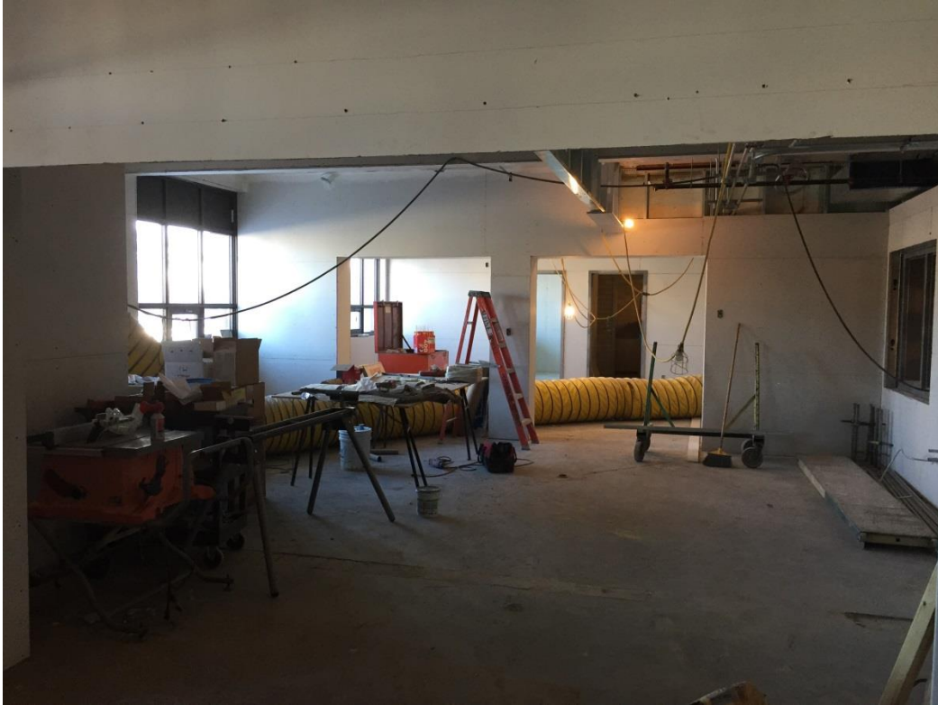
View of the original office opened up for joint reception / work area
