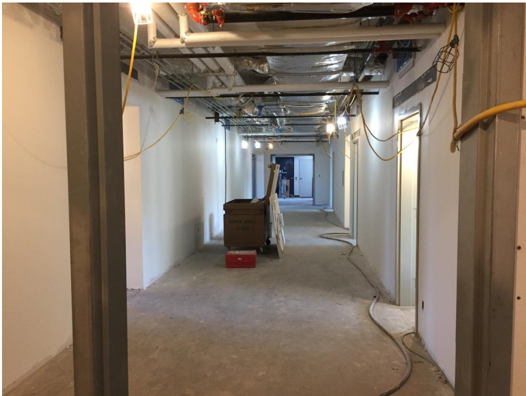
Lower hallway looking east shows completed boarding, joint filling and primer coat
